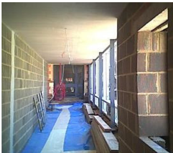
The new cloister linking the Reception area with the new guest facilities. The doors at the end used to lead into the small conference room.
