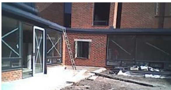
The guest courtyard; the guest refectory is on the left, the entrance cloister at the rear with the lift shaft and stairwell above.
