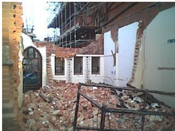
The section of cloister and print room being demolished to make room for the service road and to separate the properties.
