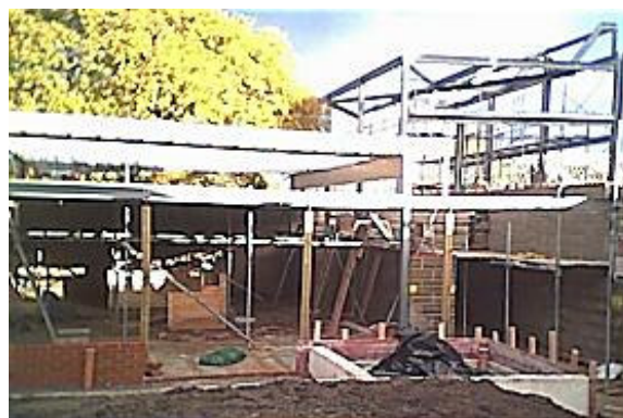
The frame for the new guest refectory. Behind can be seen the oak tree, which has been carefully preserved.
