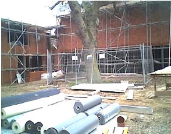
The new monastic refectory rises behind the oak tree; on the left will be the new conference rooms and guest chapel.
