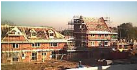
The houses on the site on the former laboratories and the Art Department.
