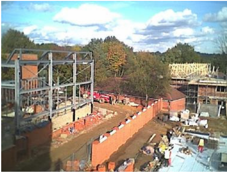
The frame of the monastic refectory was erected in October: through it the end of the existing monastery south block can be seen. The wall in the centre will be the division between monastery property and the housing development. In the foreground can be seen the roof of the underground carpark, and houses under construction lie beyond on the site of the school science block. The photo was taken from the top of the 'Ark' building.
