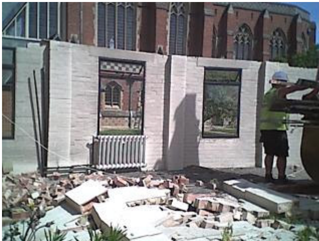
The last wall of the temporary cloister link about to be demolished.
